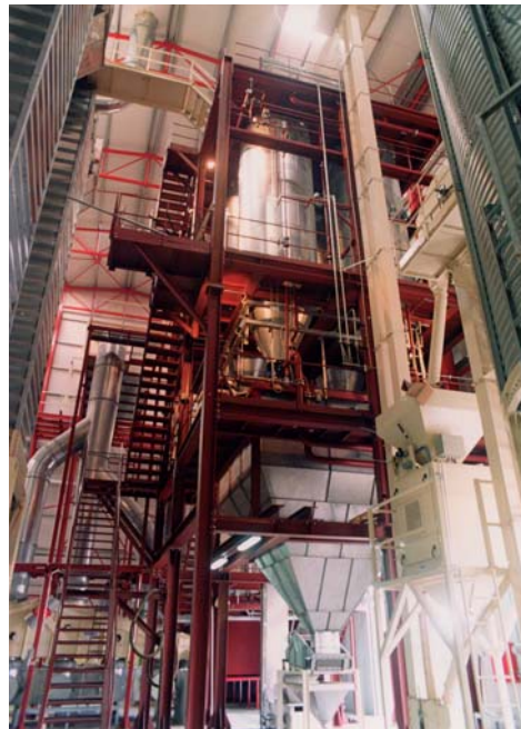
7,5 t/h parboiling plant
